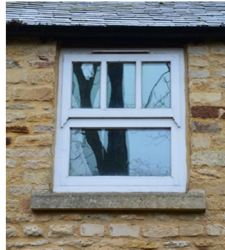
Unsympathetic UPVC window with inappropriate detailing
